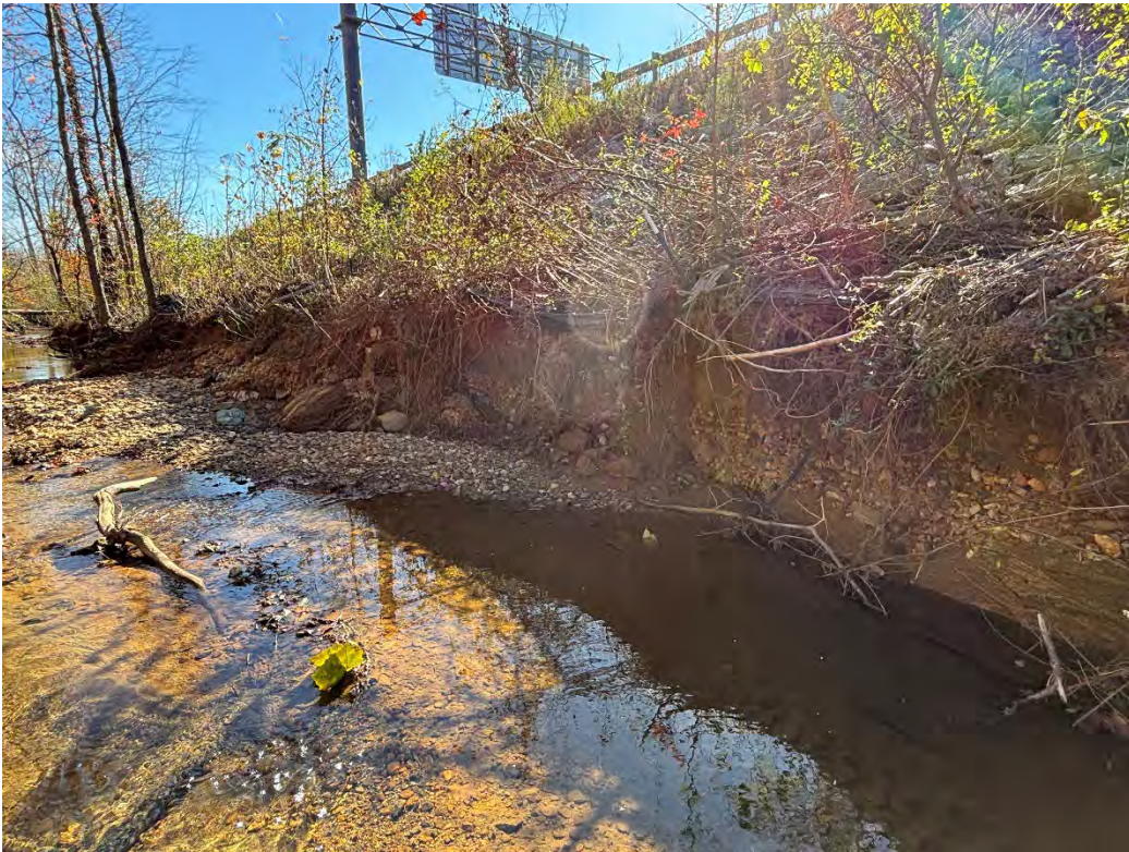
Looking Downstream into Transition Zone Streambank Erosion – November 2024
